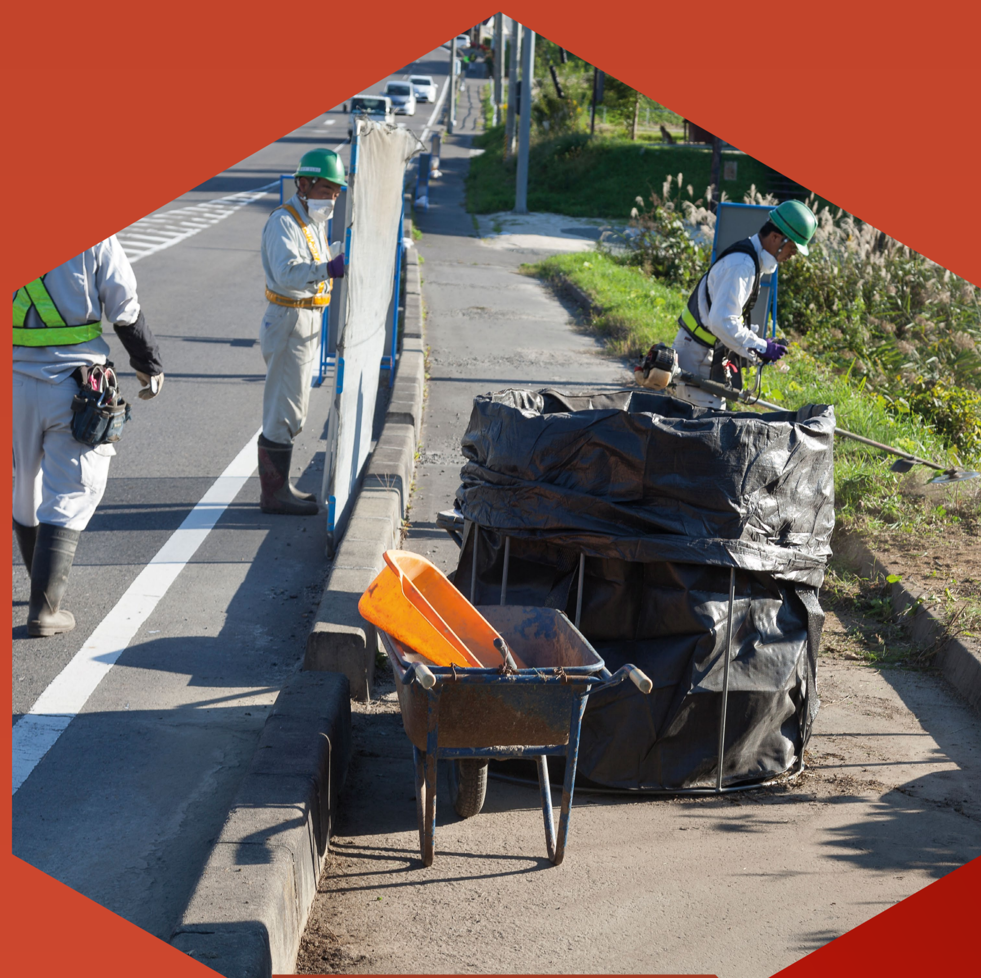
5 years after the accident, decontamination work on the Wide Area Farm road in Fukushima Prefecture.
