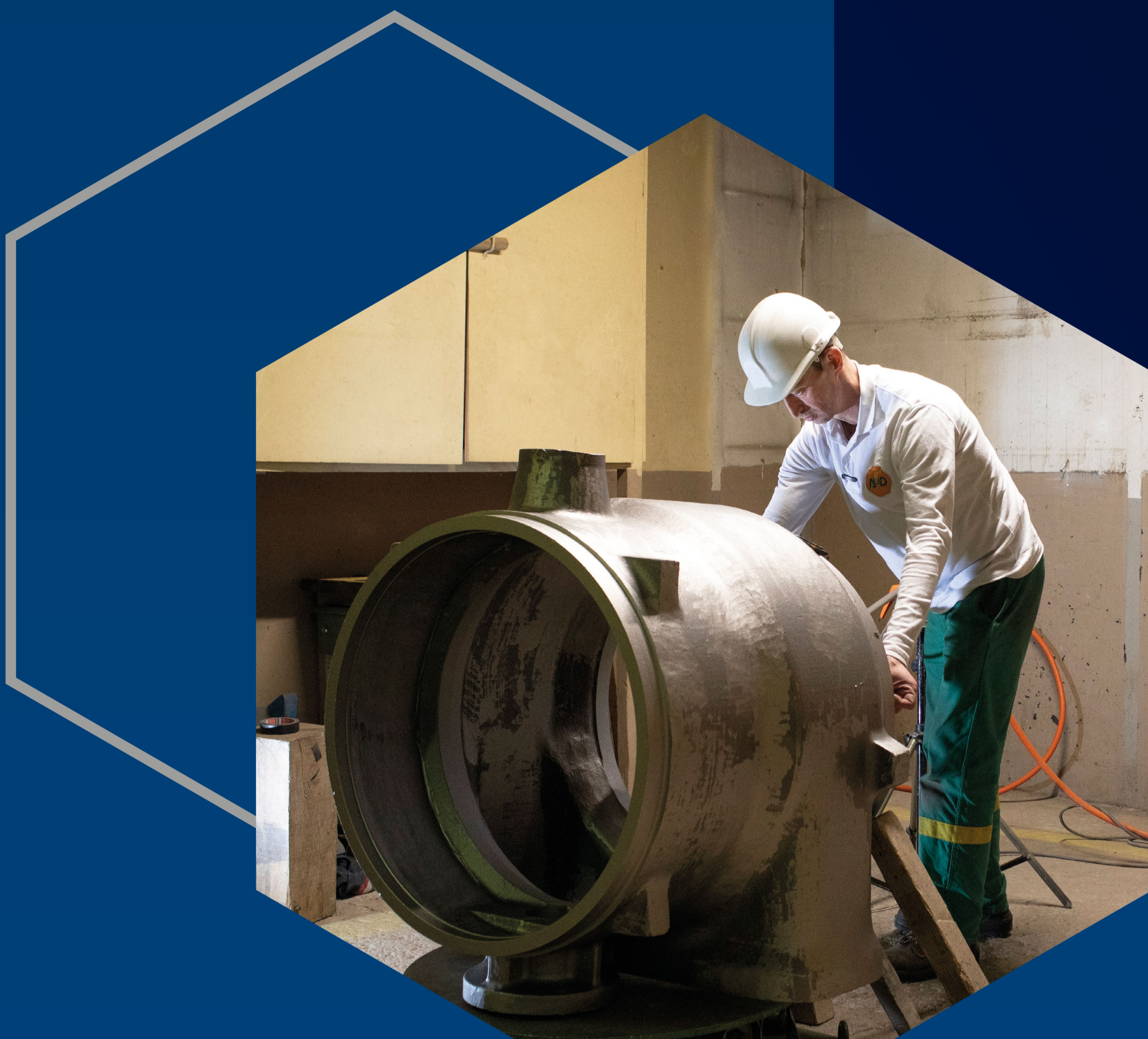
A technician prepares a gamma radiography machine to inspect a heavy piece of boilerwork. He has been specifically trained and will move away when the radiograph is triggered.
