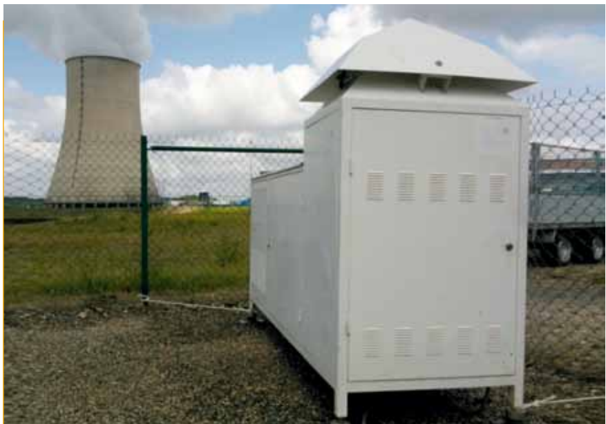
Figure IV.69 - OPERA-Air (300 m³/h) sampler installed under the prevailing winds of the Golfech NPP.
