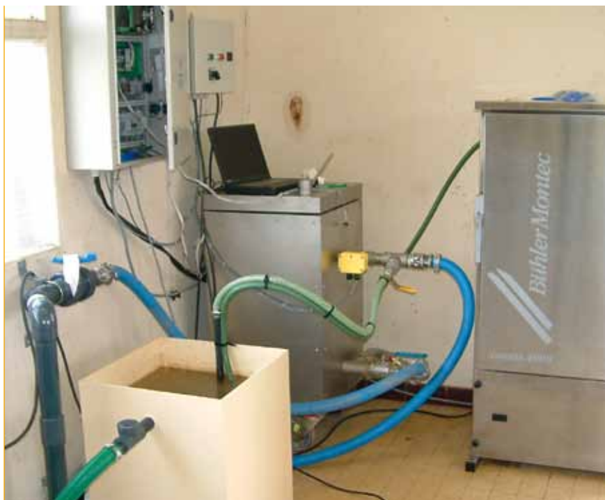
Figure IV.26 - Boé HydroTeleray station (near Agen) performing real-time radiological monitoring of water from the Garonne.
