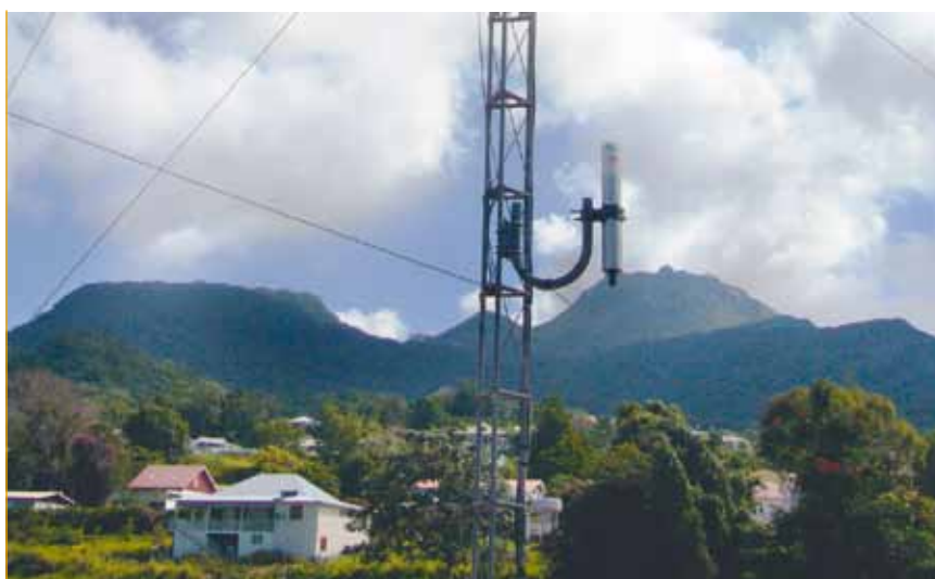
Figure IV.74 - New-generation Teleray probe installed in Saint-Claude, Guadeloupe.
