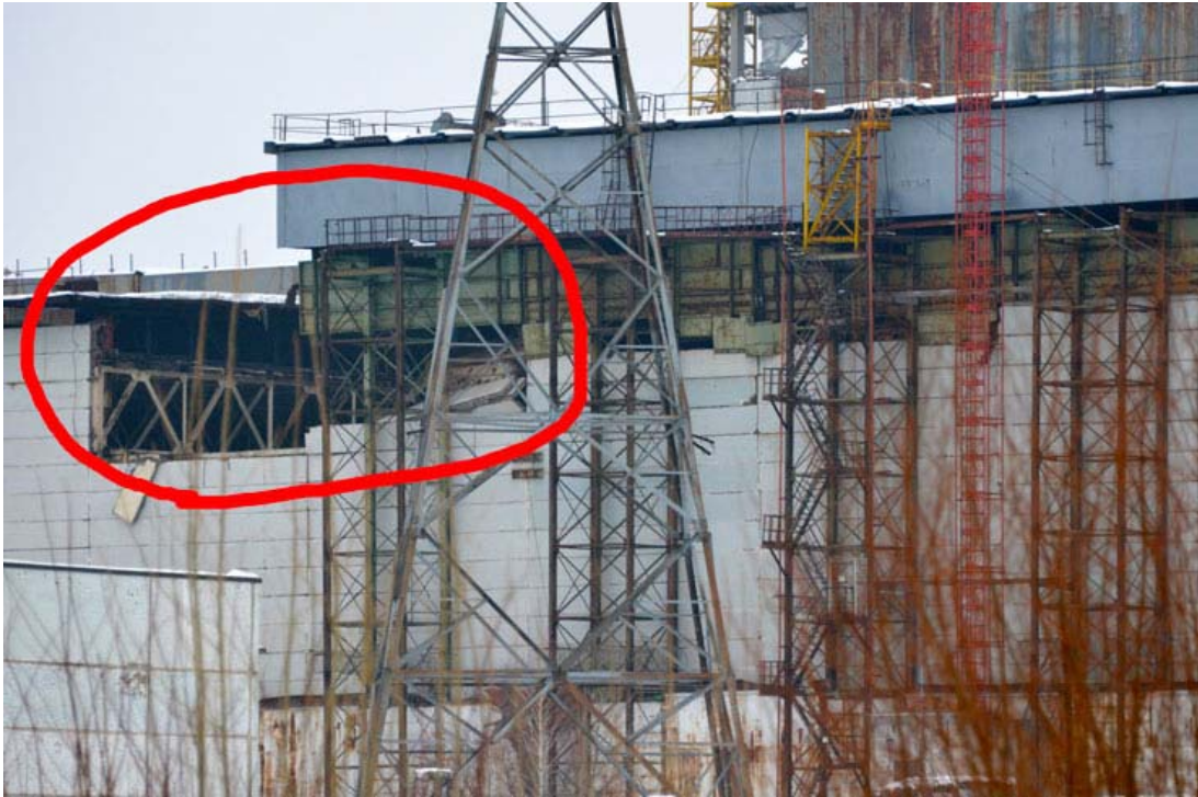
External view of the destroyed area of the turbine hall. Credits: Ukrainian Safety Authority.
