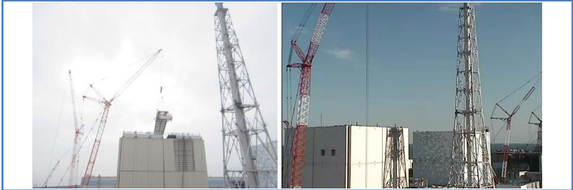
Source TEPCO - Removal of a panel of the building covering Reactor 1 (July 2015) and current condition of the building
