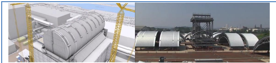
Source TEPCO - Cover of the Reactor 3 building (project plan and view of the structures before assembly)
