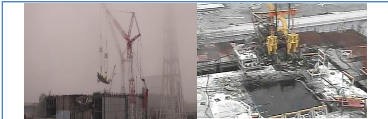
Source TEPCO - Removal of a fuel handling crane from the pool of Reactor No. 3
