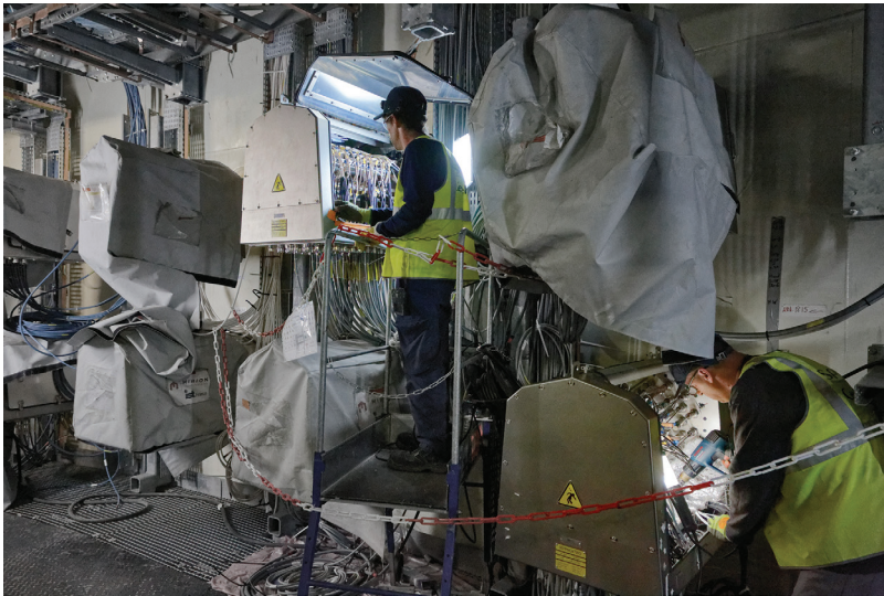
Figure 19.2. Operators inspecting electrical cables in the Flamanville 3 EPR. Alexis Morin/IRSN Media Library.
