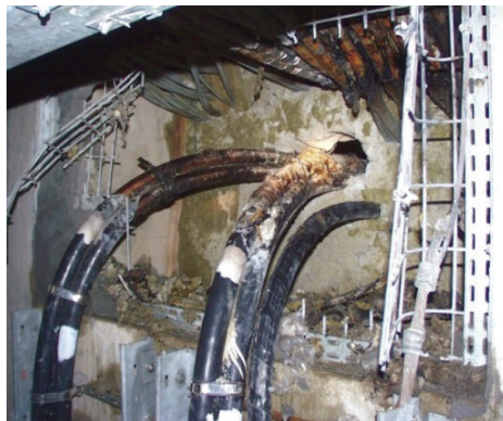
Figure 23.4. 6.6 kV cable trays after the Cattenom-2 event on 16 May 2004. EDF.
