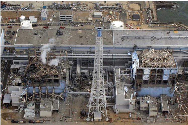
Figure 36.7. Photograph showing the destroyed superstructures of Fukushima Daiichi nuclear power plant units after the explosions. HO/AIR PHOTO SERVICE/AFP.
